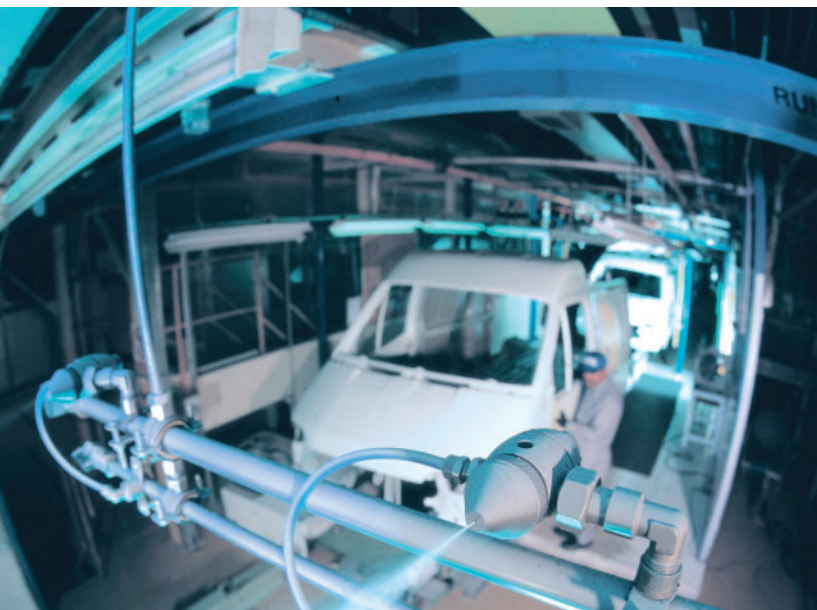
Humidification in an automotive painting plant
